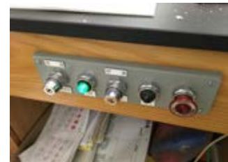
Science Room Gas Shutoff
