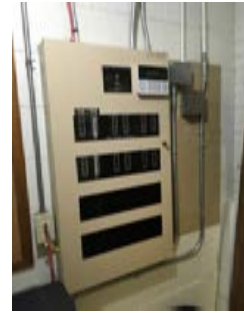
Fire Alarm Control Panel
