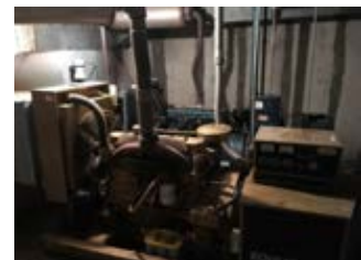
Old Generator Set
