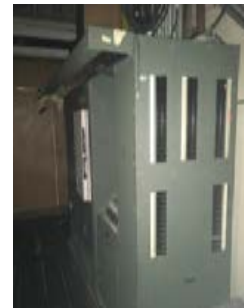
Theatrical Dimmer Rack
