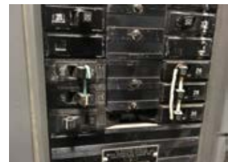
Single Pole Breaker Fire Hazard
