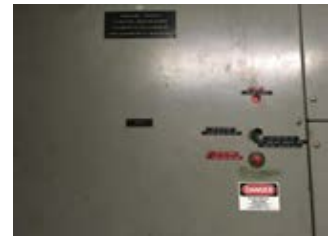
Main Electric Service
