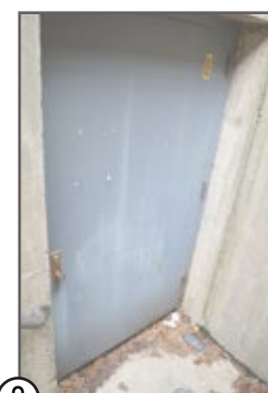
⑧ HOLLOW METAL DOOR & HOLLOW METAL FRAME, STAFF INDICATED SCHEDULED FOR REPLACEMENT
